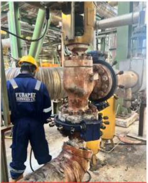
AFTER ONLINE LEAK DEALING
