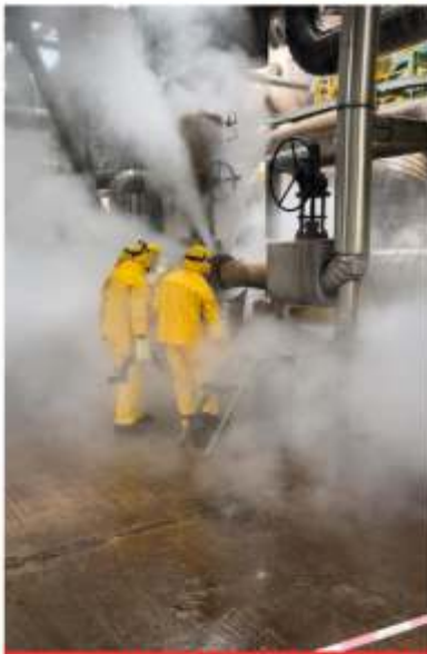
BEFORE ONLINE LEAK SEALING
