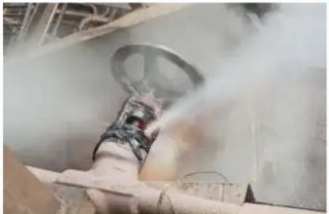
VALVE GLAND LEAKAGE
